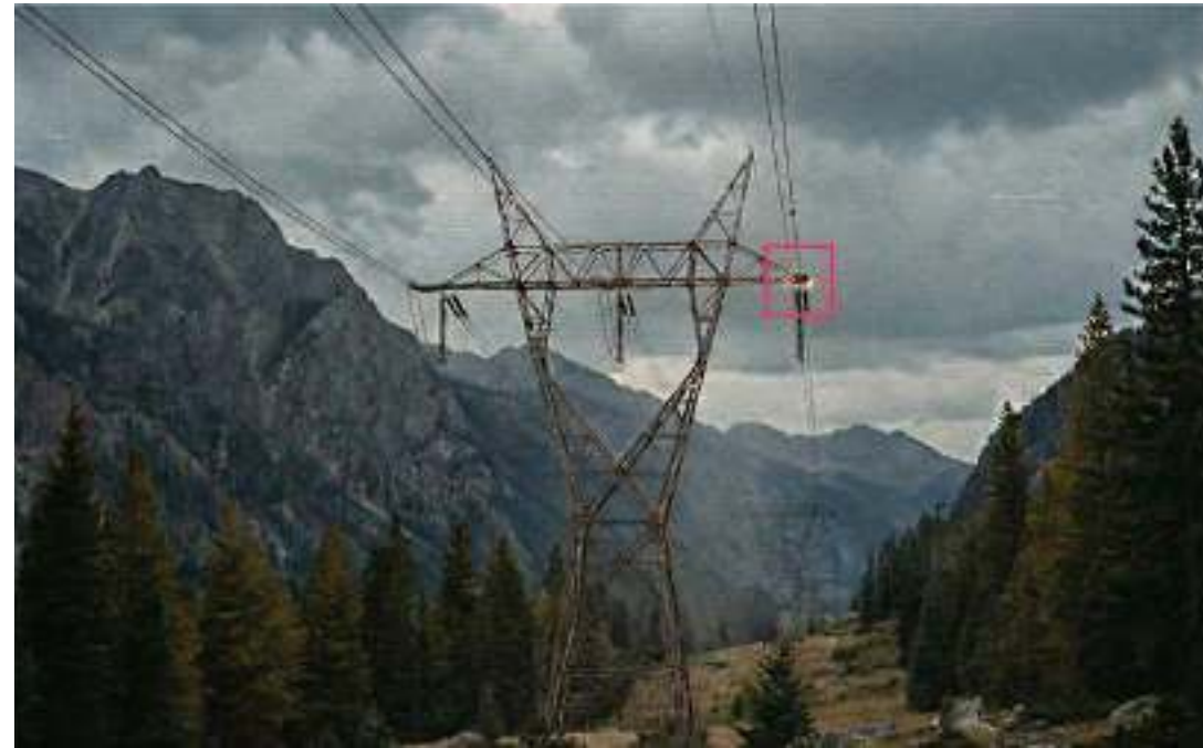
Equipment spark detection
