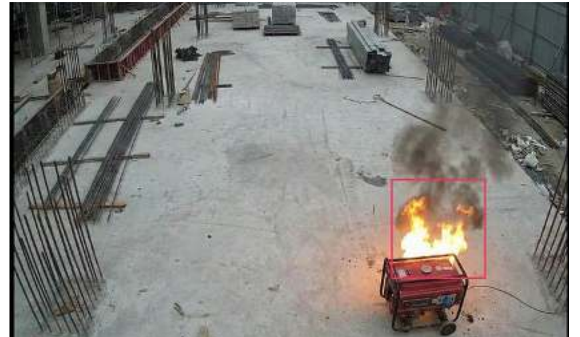
Equipment catching fire
